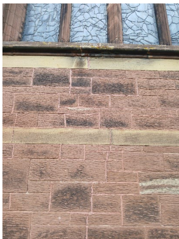
Crack beneath west window
