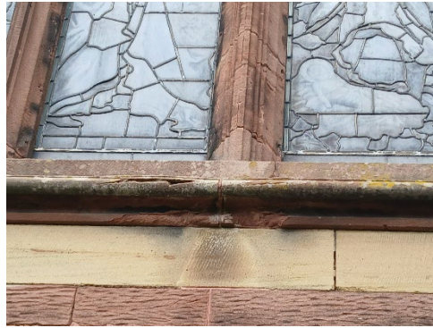
Decay to stone cill moulding below west window
