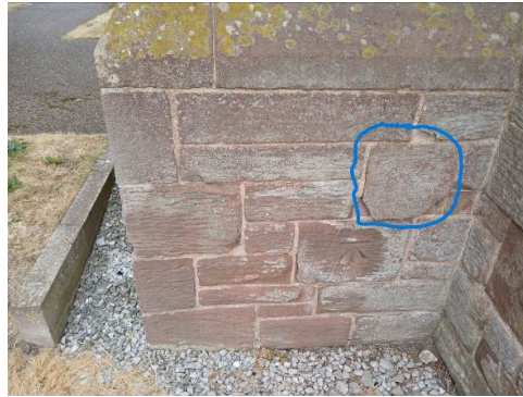
Example of delaminated loose face to stone
