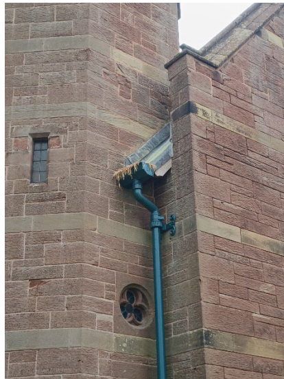
Newly decorated rainwater goods, blocked gutter
