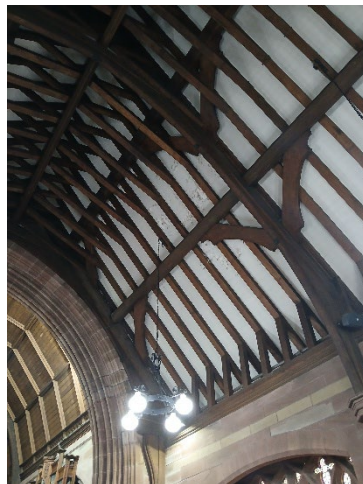
Flaking paint to ceiling over nave
