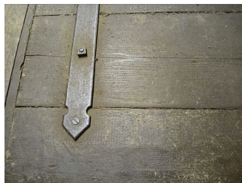
Woodworm/furniture beetle damage assumed no longer active
