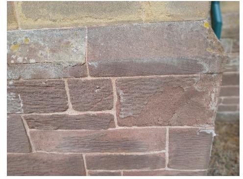
Example of delaminated face to stone
