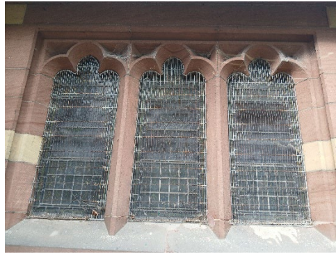
Corroded security grille
