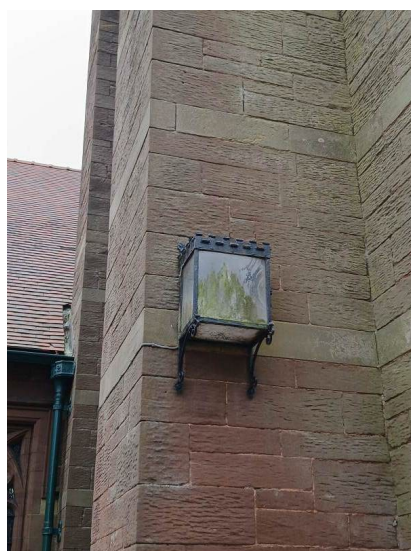
Light fitting requiring redecoration.
