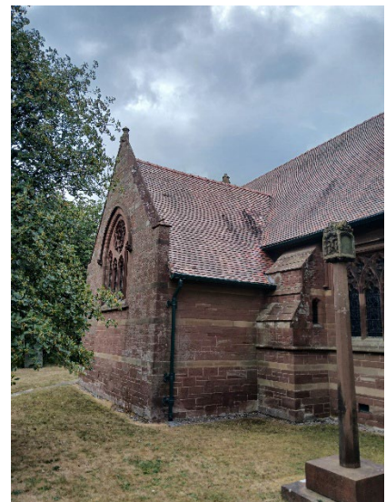
Two slipped and two broken roof tiles to west roof slope of the north transept
