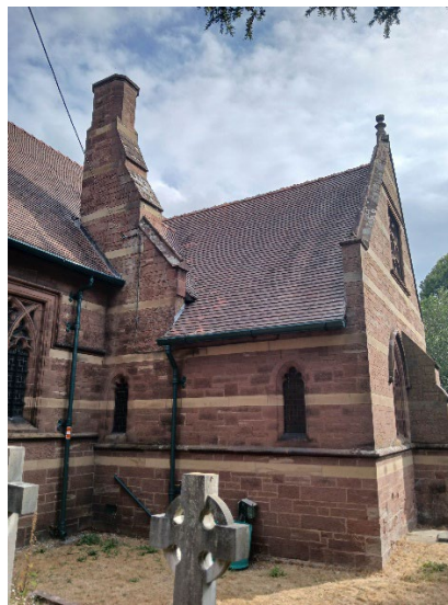
Two slipped tiles and broken tile to west roof slope of the south transept
