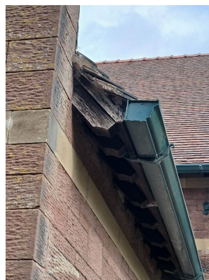
End rafters requiring re-staining for protection
